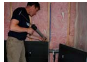
A continuous 1/2" bead of wedi joint sealant is applied on the foam edges of a wedi building panel before another panel is joined butted tightly.
