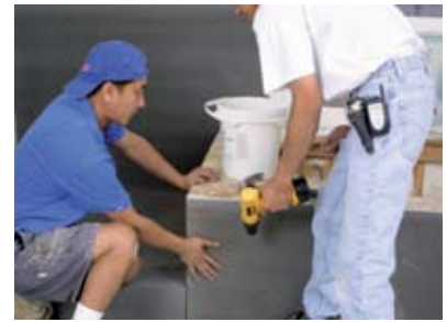
On solid backing constructions use a modified mortar and wedi fasteners to apply wedi building panel.
