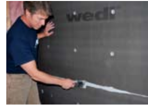
All excess wedi sealant is spread flat over all joints using a putty knife. Where needed, an extra bead of sealant is applied on top of the joints and spread flat. The joints should be covered a full 3/4" on both sides of the seam.
